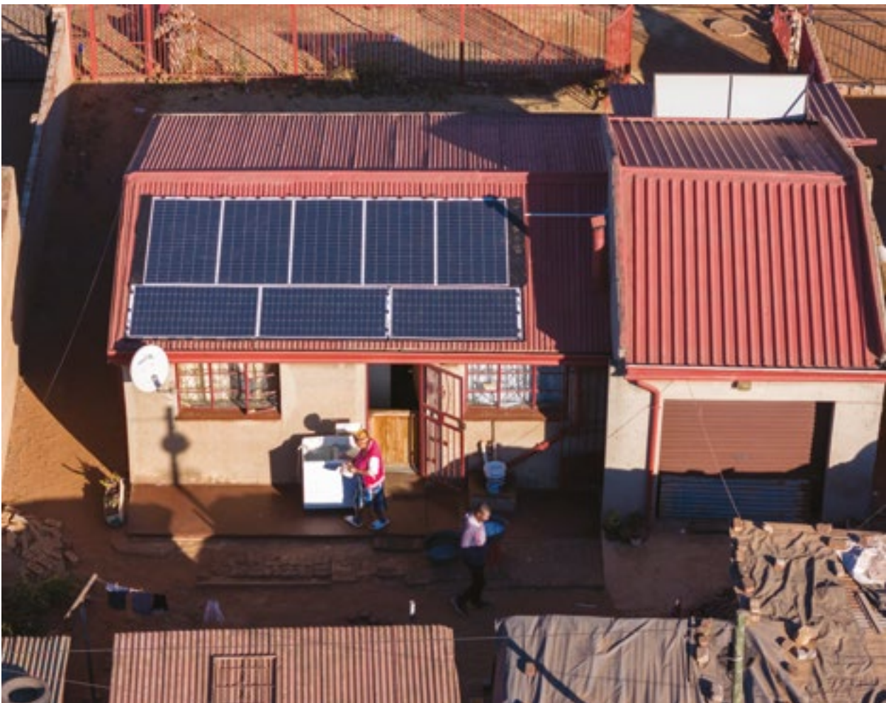
Installed Wetility solar
