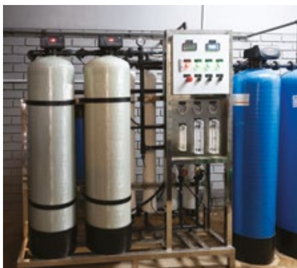
Water purification system
